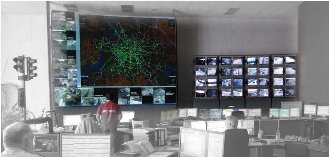
Figure 2.3: Traffic Management Center Headquarters Berlin - provided by [208]
