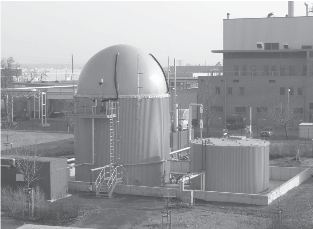
Figure 4 The GICON percolate fermentation plant at the RABA Erfurt Ost mechanical and biological waste treatment facility.
