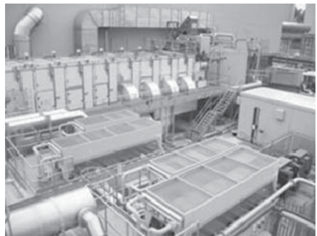
Figure 3 Bredbury Parkway Digestate Dryer
