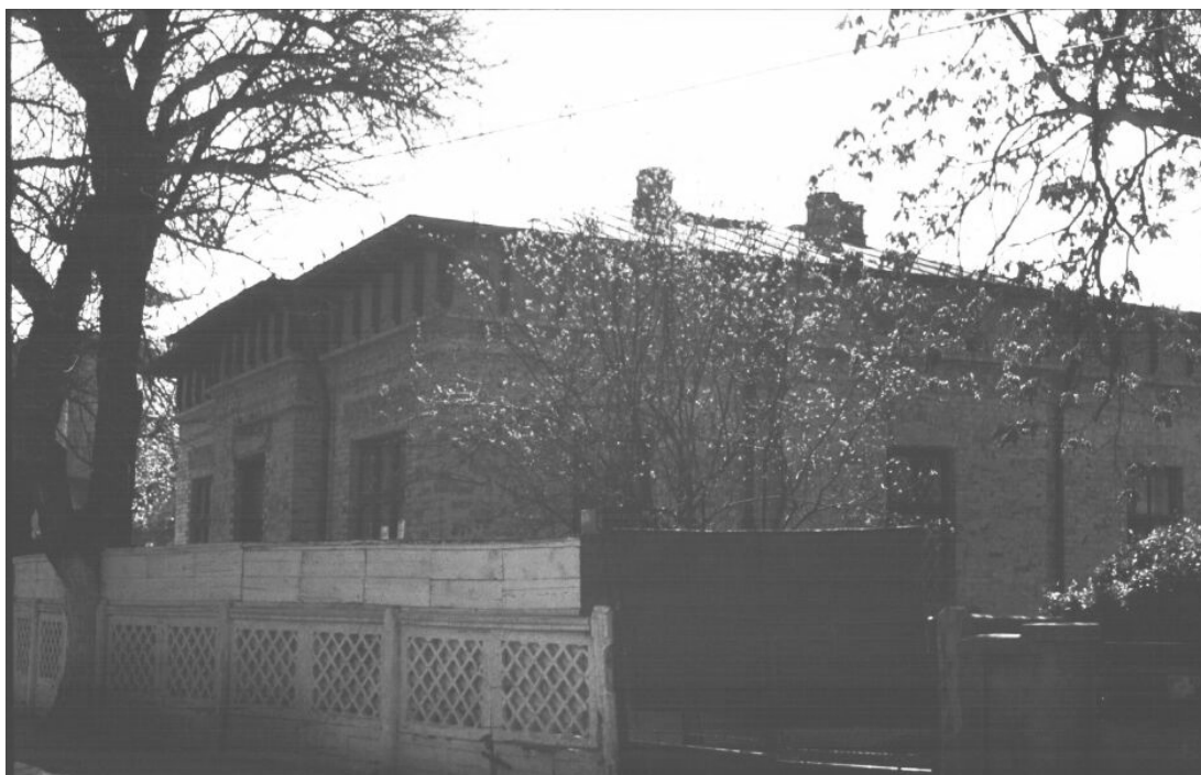
Figure 4-31: Damage at corner. Photo by Maria Bostenaru, 2002.
