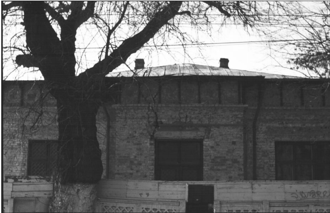
Figure 4-30: Damage over opening (from Bostenaru, 2004, TAFEL VII)
