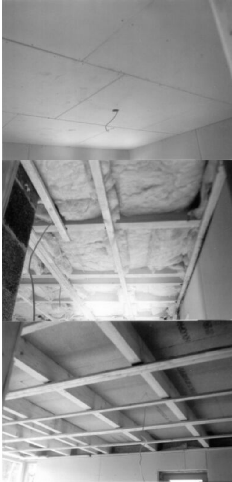
Figure 2-21: Construction details of floors (new building): from bottom to top different steps in finishing. Photos by Maria Bostenaru, 1998.
