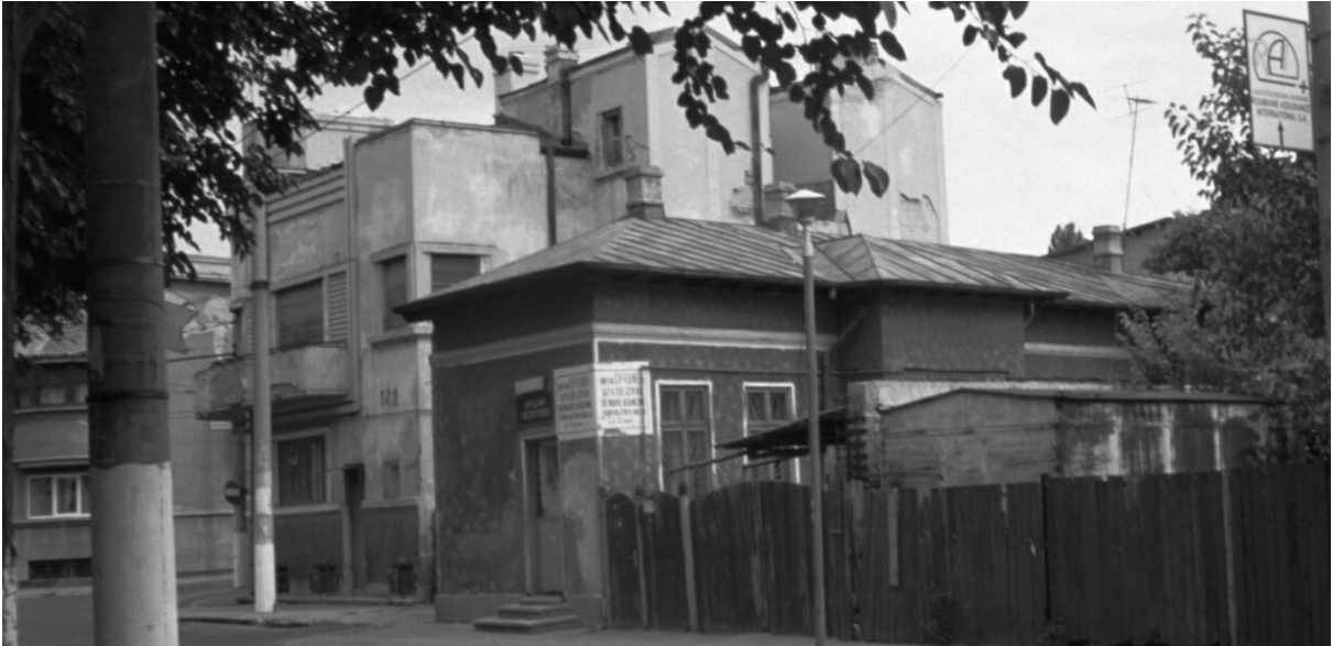
Figure 4-9: Structural modification: one closed facade window and one changed to door opening. Photo by Maria Bostenaru, 2002.
