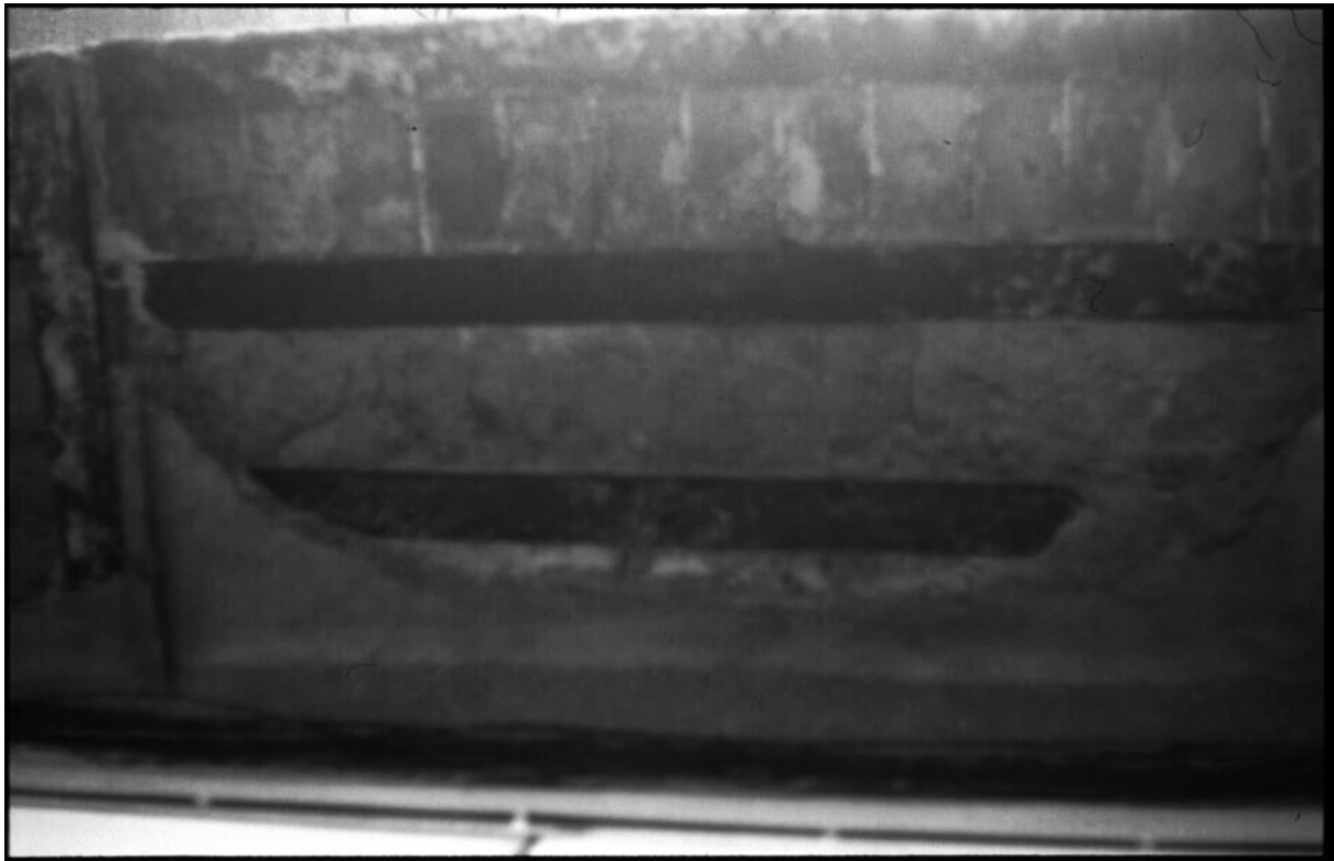
Figure 4-28: Photo of a brick and metal joists floor structure. Photo by Maria Bostenaru, 2002.
