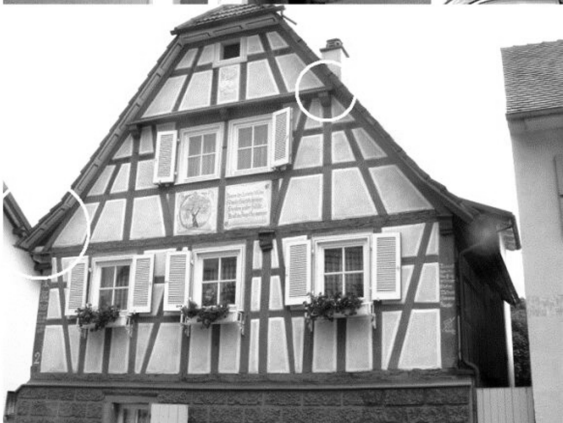
Figure 2-18: Connection between horizontal and vertical load bearing elements: side wall (top) and typical gable solution (bottom). Photos by Michael Kauffmann, 2004.
