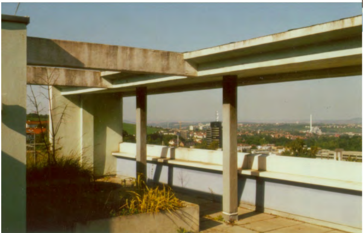
Figure 3-18: Details showing the way horizontal and vertical (iron)reinforced concrete and vertical metal elements are combined in Le Corbusier's building in Stuttgart Weissenhof. Photos by Maria Bostenaru, 2002.
