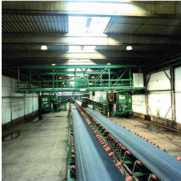
Abbildung 3 MBT plant of Ennigerloh, intensive decomposition hall of BIOWEST
