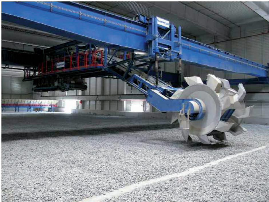
Picture 6: TAIM WESER "ROTOPALA"-Windrow-Turner (Ready for Hot-Start-Up)
