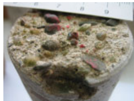
Figure 7: Example of corrosion with abrasion showing protruding particles and surface cavities
