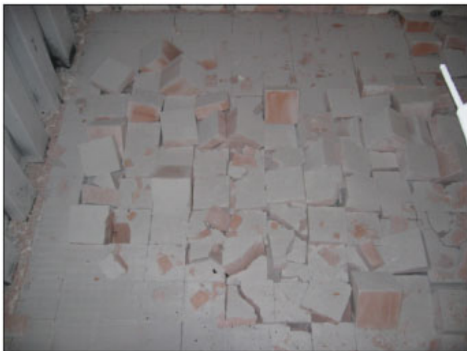
Figure 2: Siloxane problems in RTO plants, destroyed heat exchangers
