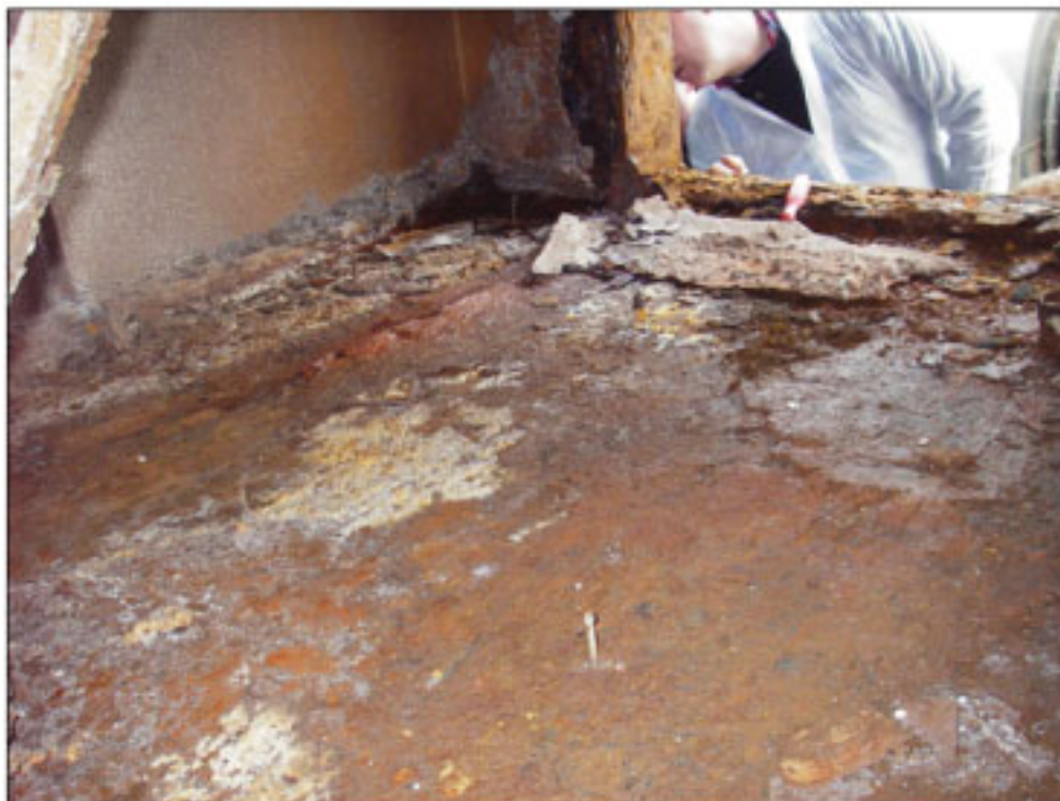
Figure 4: Corrosion in the dirty gas canal
