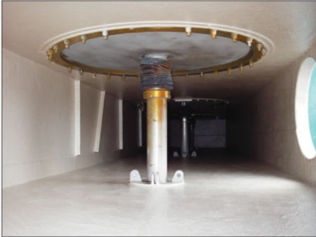
Figure 5: Re-engineered dirty gas canal
