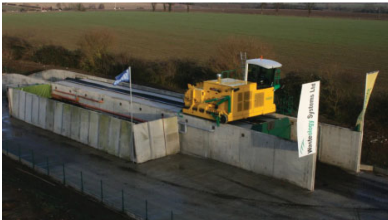
Figure 4: Dynamic Tunnel Composting – view of the pilot site
