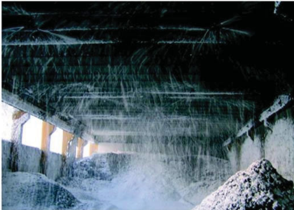
ONE SEVEN Extinction system for automatic fire fighting in a storage hall for recycling products
