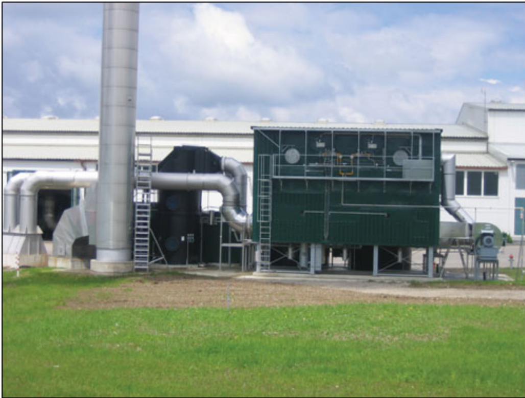
Figure 1: RTO plant with scrubber
